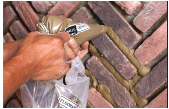
Even though Eldorado Brick is being grouted in this picture, the theory is comparable when grouting Eldorado Stone.
